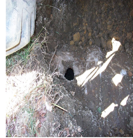
Illegal Tap Into Stormwater System – Sink And Dishwater Discharge
