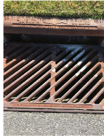
Paint Washout In Catch Basin
