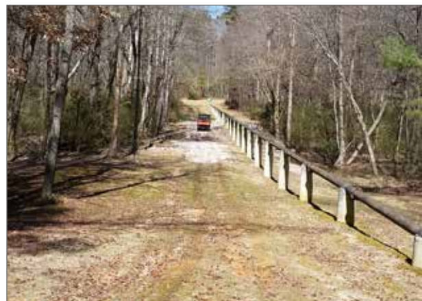
Field Investigations - Little Creek Sewer Easement to Five County Stadium behind Zebulon Community Park
