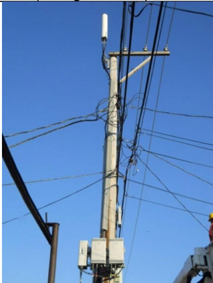
Typical placement on an electrical utility pole
