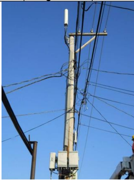
Typical placement on an electrical utility pole
